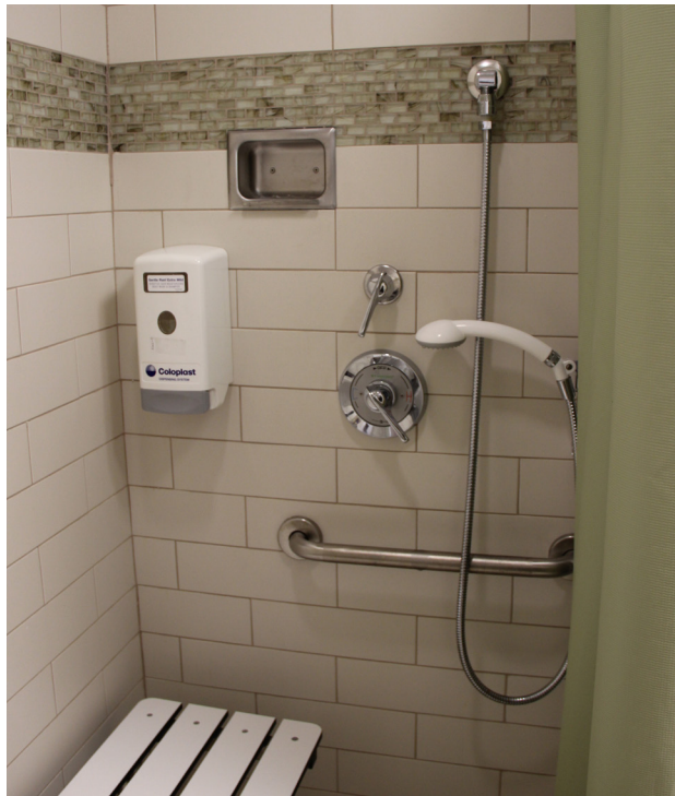
Figure 15 Lawrence + Memorial Hospital (US) - New Unit Shower in new unit
