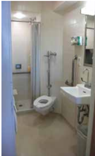
PICTURE 5 Bathroom with no grab-bars accessible to the toilet
